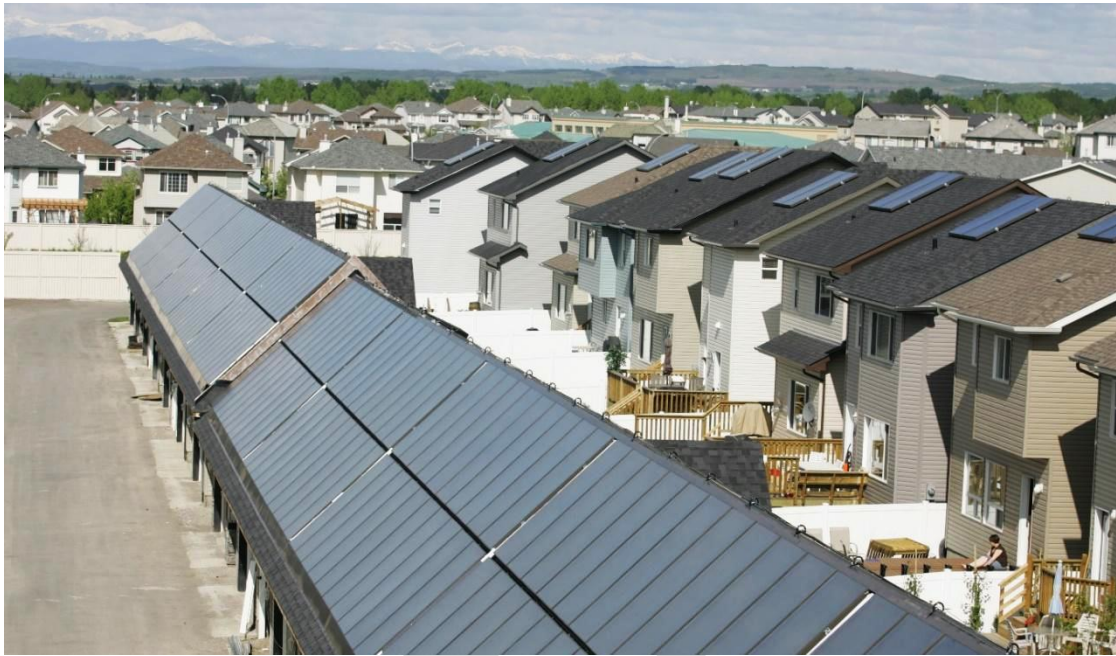
Figure 5: View of houses and adjoined garages equipped with rooftop solar thermal collectors for hot water and space heating, respectively.
